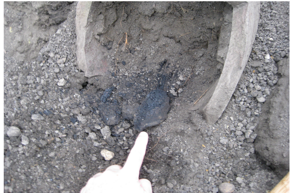
Coal-tar that has seeped out from the toxic pipe.
